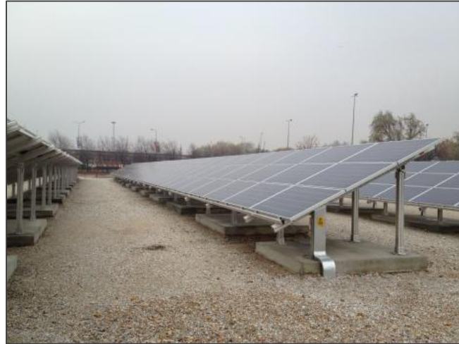
Figure 4-3 PV Panels and Holders
